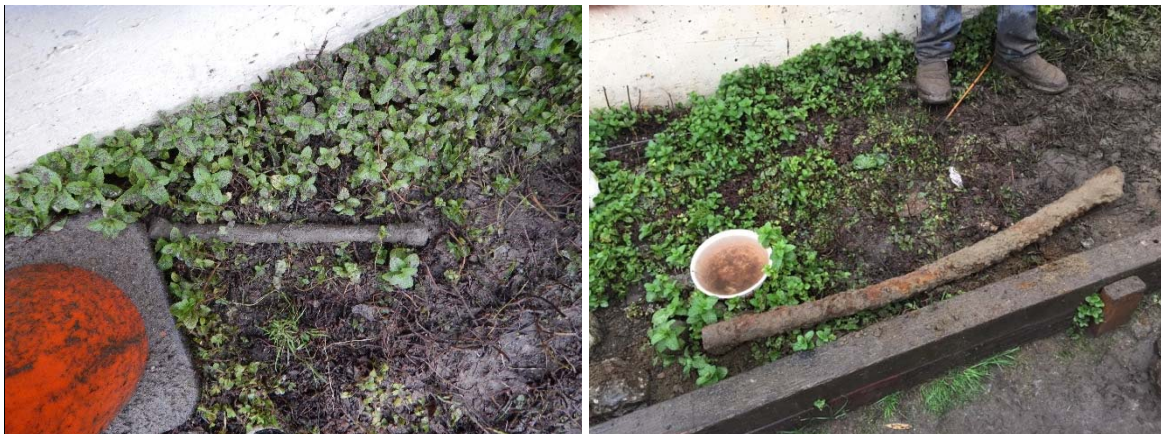
Photograph 8: Loose pipes discovered within the excavation area, the first being approximately 1.0 feet in length and the second 4.0 feet in length.
