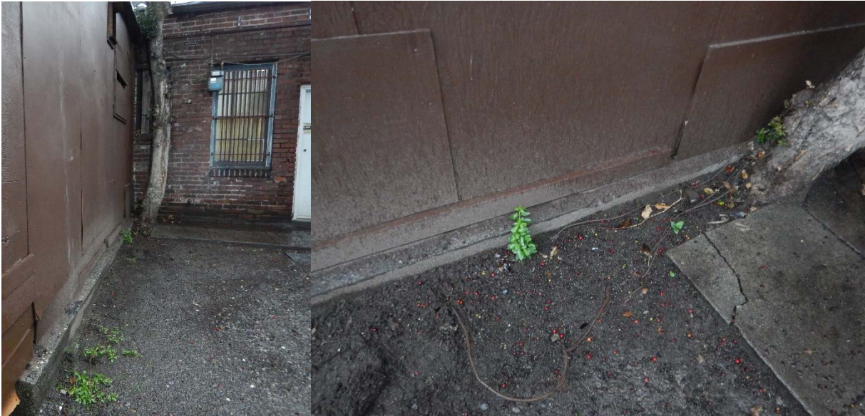
Photograph 3: Southern border of the Building Addition, facing east, showing wiring identified by the utility locator to be conductively grounded to the same location as the three pipes. The wiring led from the window behind the tree pictured, and continued below ground and potentially beneath the Building Addition.
