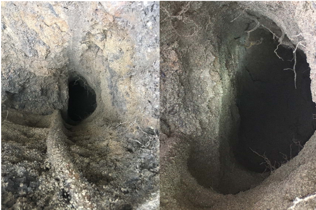
Photograph 6: View along Pipe 3 and the eastern sidewall of the tank. The tank was determined to be 4.5 feet in height. The excavation reached approximately 8 feet bgs and no groundwater or petroleum impacted soil were observed.
