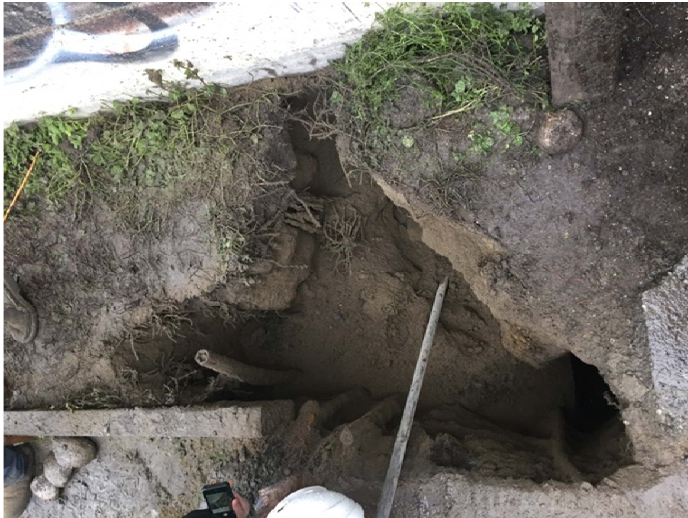
Photograph 7: View of total extent of the excavation, with the Jurgensen building retaining wall in view.
