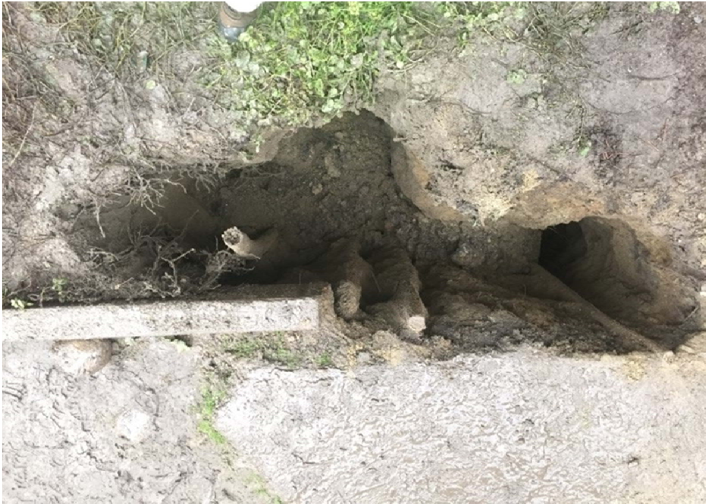
Photograph 5: Excavation in progress with four pipes and steel tank surface in view approximately 3.3 feet bgs (Pipe 1 on the far-left [west], followed by Pipe 4, Pipe 2, and Pipe 3). The tank was observed to be cylindrical and have a diameter of approximately 4.0 feet.
