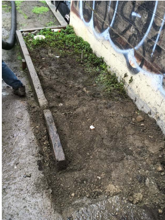
Photograph 13: View of the excavation area after backfilling, facing west-northwest. Field screening did not indicate the presence of petroleum-impacted materials; therefore, the excavated soil was backfilled into the excavated area.
