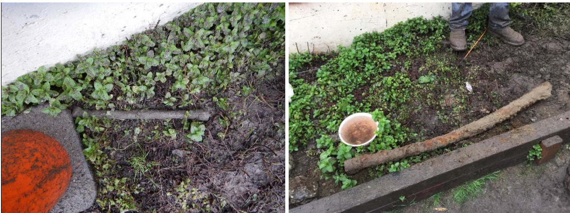
Photograph 8: Loose pipes discovered within the excavation area, the first being approximately 1.0 feet in length and the second 4.0 feet in length.
