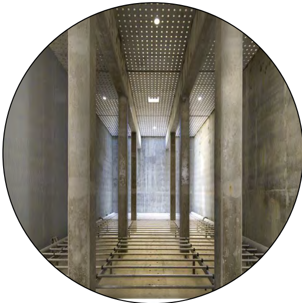
Interior of BIOSTYR Cell
