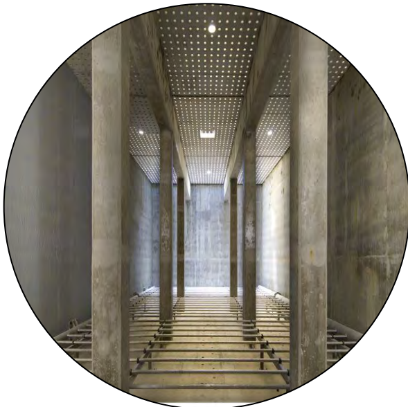
Interior of BIOSTYR Cell
