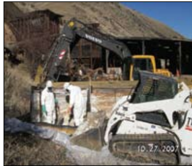
Cleanup of an Idaho mine near the Salmon River (photo courtesy of EPA)
