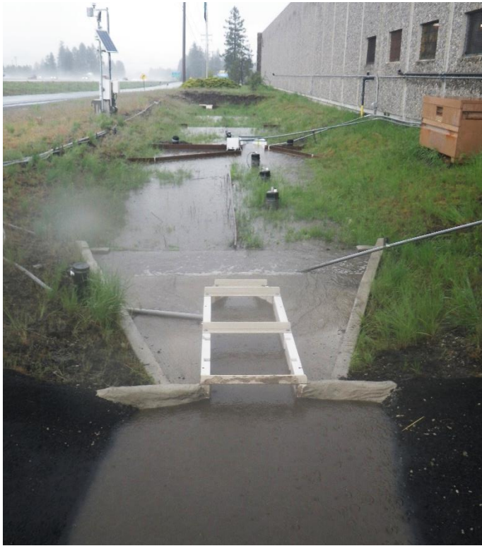
Figure 4. Example of a compost-amended biofiltration swale. Stormwater is filtered as it flows along the grass in the swale and infiltrates into the topsoil and compost. Photo: Washington State Department of Transportation.
