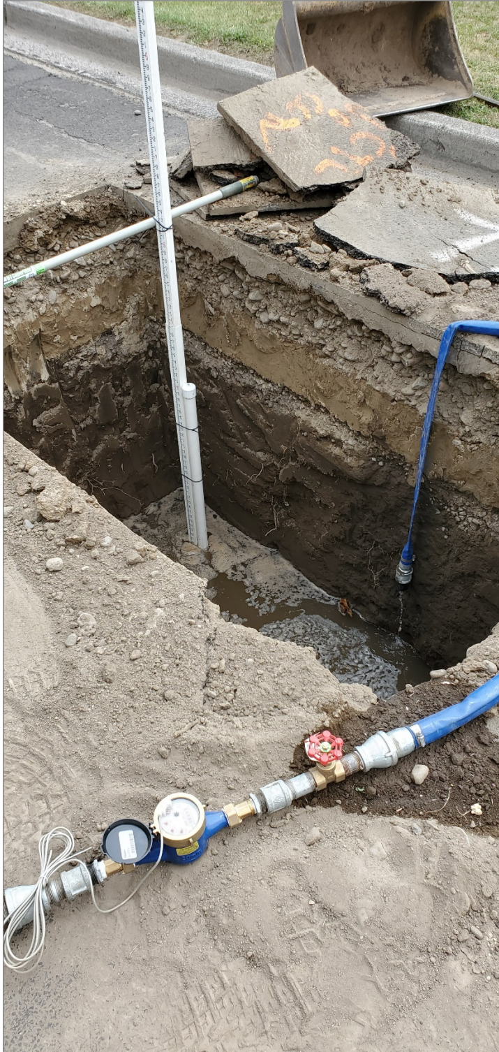
Photograph 4. INF #2 small-scale PIT. (July 20, 2021)
