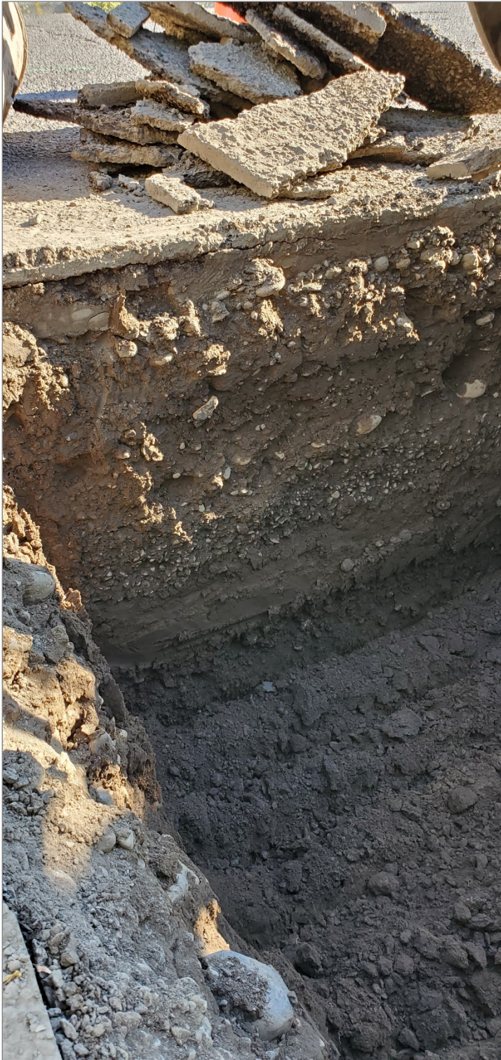
Photograph 1. INF #1 small-scale PIT. (July 22, 2021)
