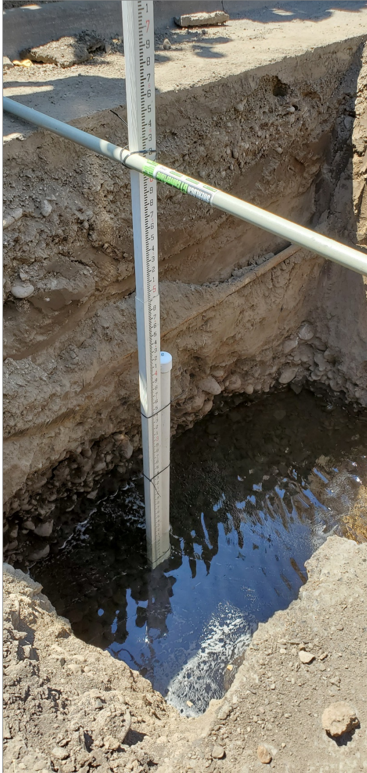
Photograph 2. INF #1 small-scale PIT. (July 22, 2021)
