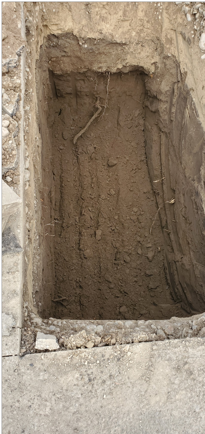
Photograph 3. INF #2 small-scale PIT. (July 20, 2021)
