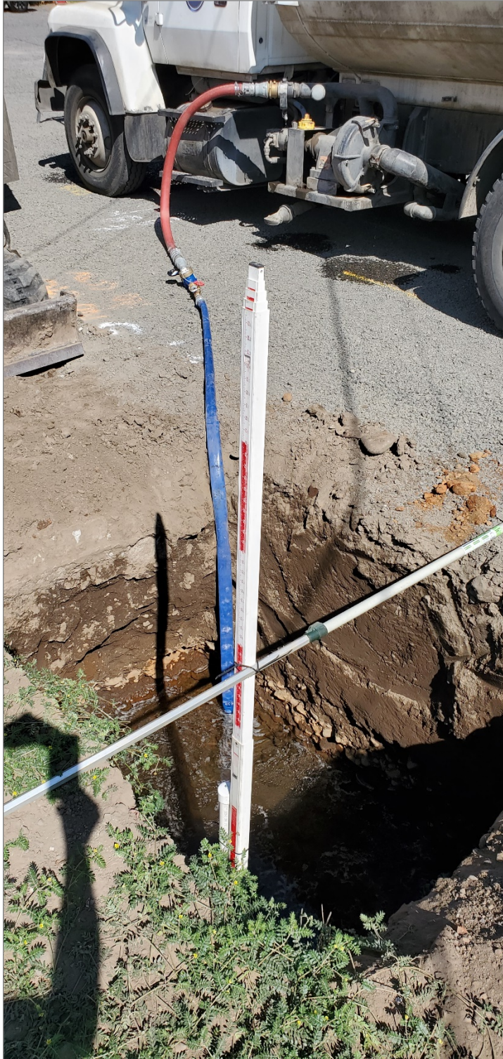
Photograph 6. INF #3 small-scale PIT. (July 23, 2021)
