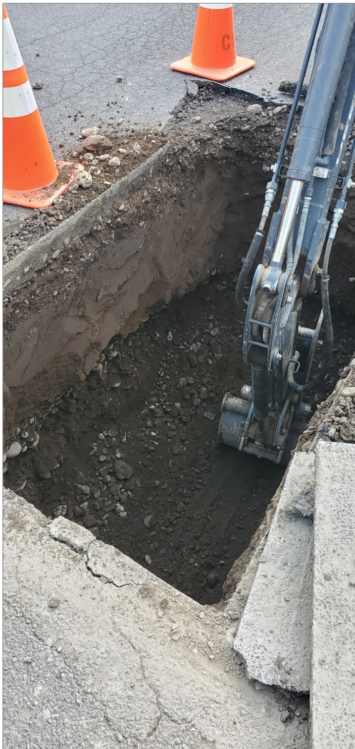
Photograph 7. INF #4 small-scale PIT. (July 21, 2021)
