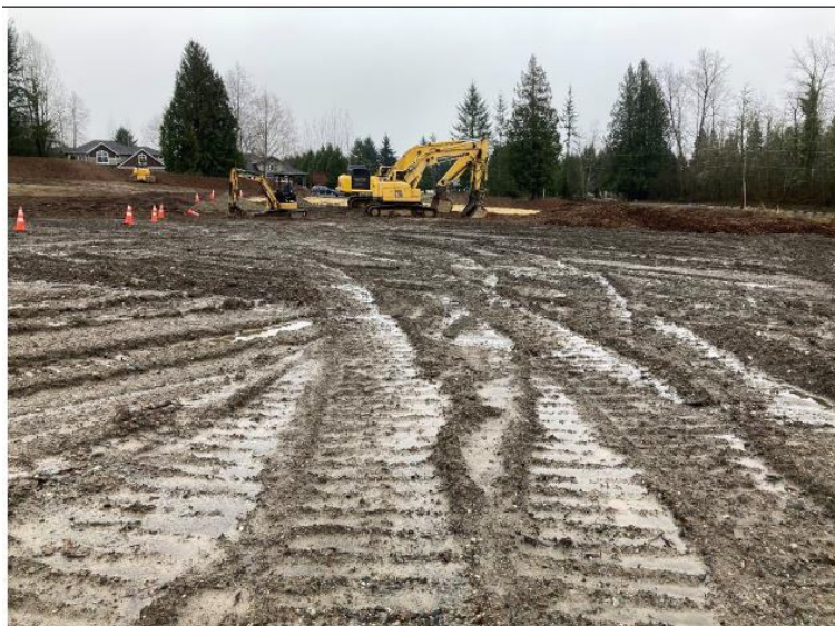
Figure 1 Edelbrock Horse Corral is actually an unlicensed landfill accepting waste construction soil. The disturbed area is 8.23 acres. Photo from Ecology inspector Charles Hackel inspection report dated April 1, 2024
