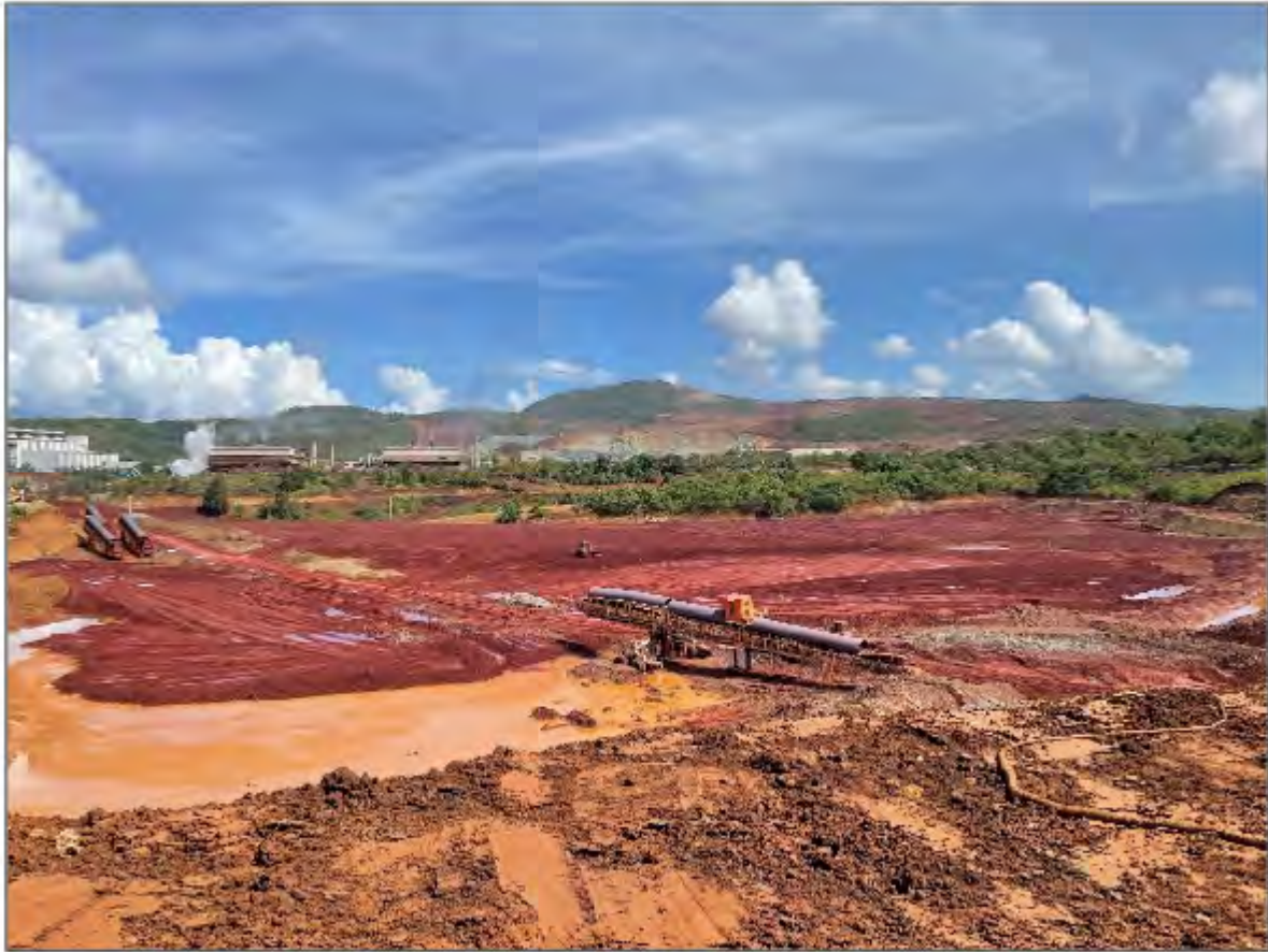
Figure 9-11: View of DSTF area with significant water ponding
