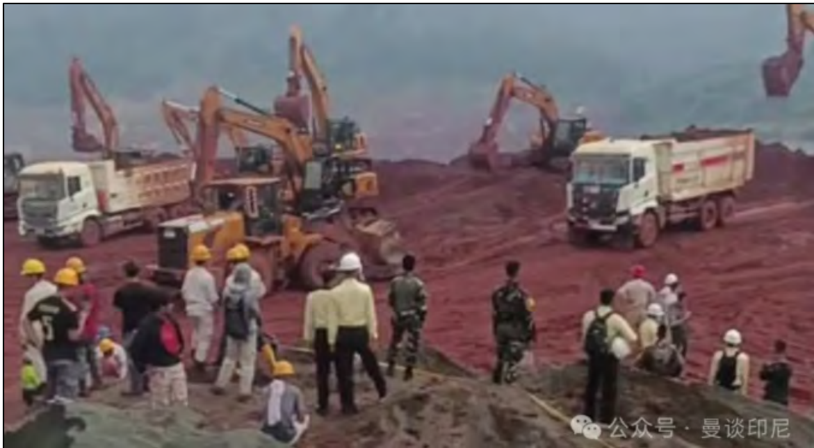
Figure 42b. On March 22, 2025, excavators search for four buried workers from the collapse on the previous day of the filtered tailings storage facility of PT Qing Mei Bang (QMB) New Energy Materials in the Indonesia Morowali Industrial Park (see Figs. 3, 23, 24, and 41a). The four workers were employees of PT Morowali Investasi Konstruksi Indonesia (MIKI), which is a contractor of PT QMB New Energy Materials. Photo from 曼谈印尼 [Man in Indonesia] (2025).
