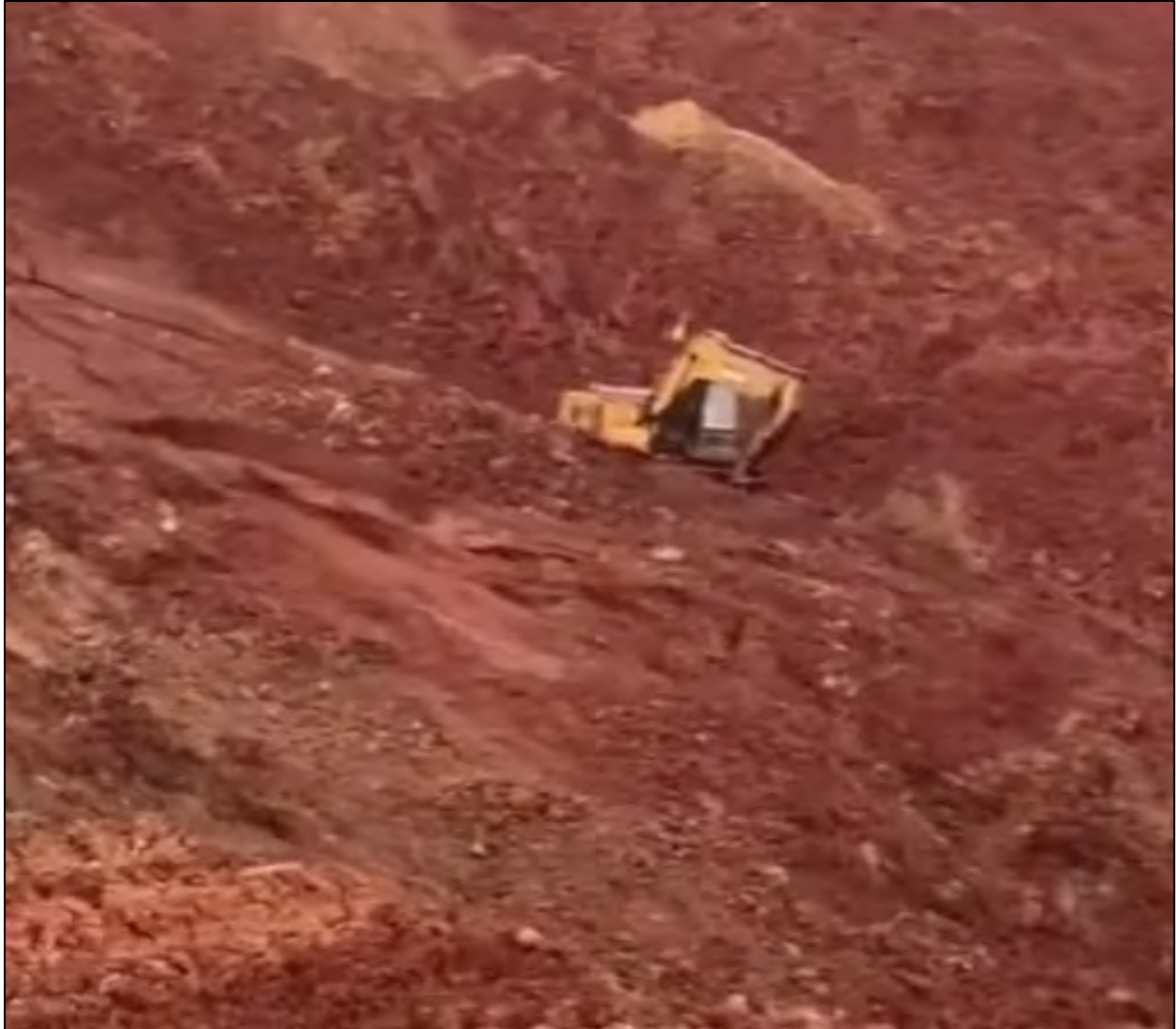
Figure 45. A bulldozer was engulfed by a landslide at a filtered tailings storage facility of the Indonesia Morowali Industrial Park (see Figs. 3 and 23) in September 2023. Still image at 0:03 from Kuli Tambang Random [Random Mineworker] (2023).
