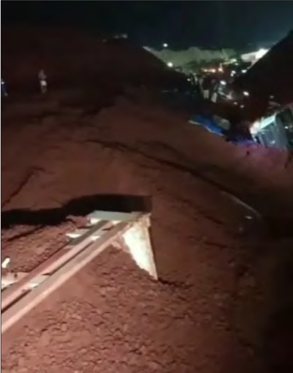
Figure 43. On March 27, 2025, an ore stockpile collapsed at the PT Qing Mei Bang (QMB) New Energy Materials project in the Indonesia Morowali Industrial Park (see Figs. 3 and 23), resulting in the burial of heavy equipment. The location of the ore stockpile is not known. Still image at 0:13 from video shared by mineworker.
