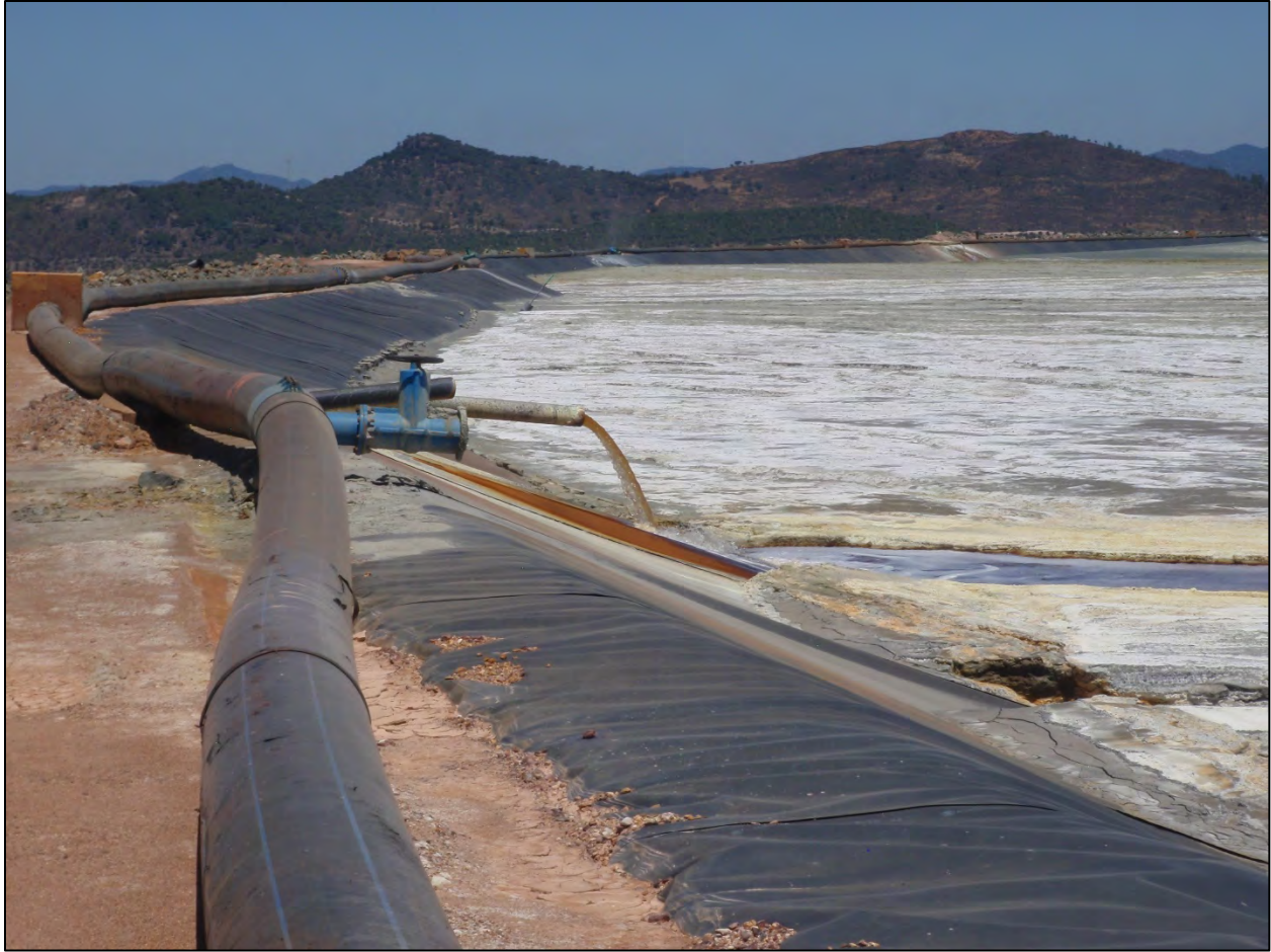
Figure 8a. A mixture of water and tailings with a solids content of 35% by mass is hydraulically discharged into the tailings pond from the crest of the Cobre dam at the Atalaya Mining Riotinto mine in Andalusia, Spain (see Fig. 7). Because of the lack of compaction, the loosely-packed tailings are susceptible to liquefaction (see Fig. 10). Photo taken by the author on June 21, 2019.
