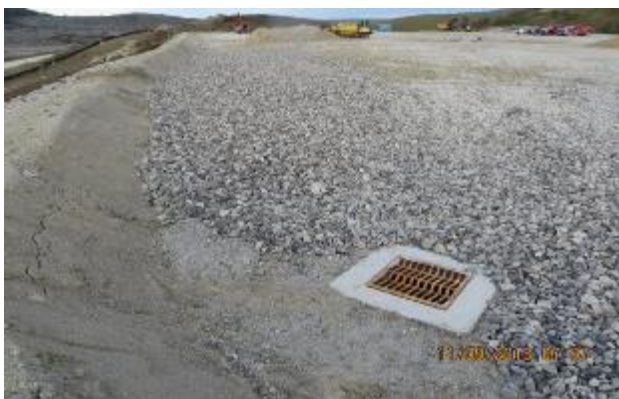
Rip Rap Apron around Catch Basin
