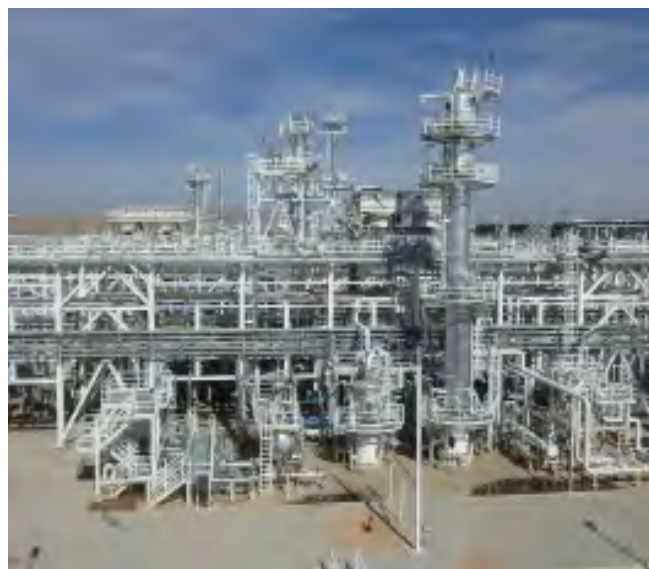
Natural gas processing plant
