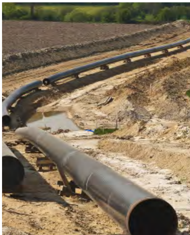
Natural gas transmission lines
