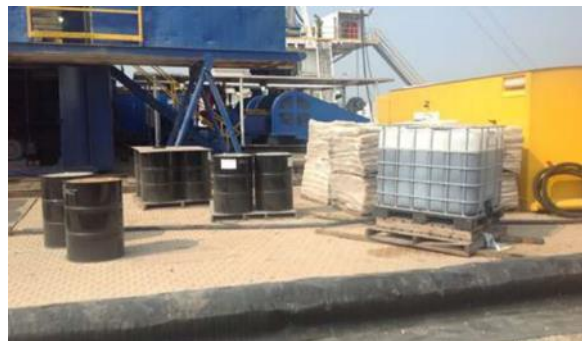
Frac Chemicals in 2 nd Containment
