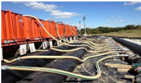
Frac Tanks / Manifold in 2 nd Containment
