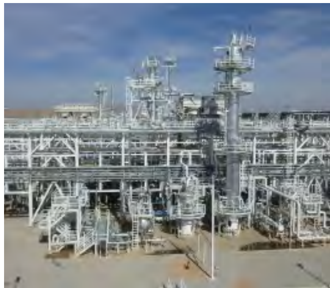
Natural gas processing plant
