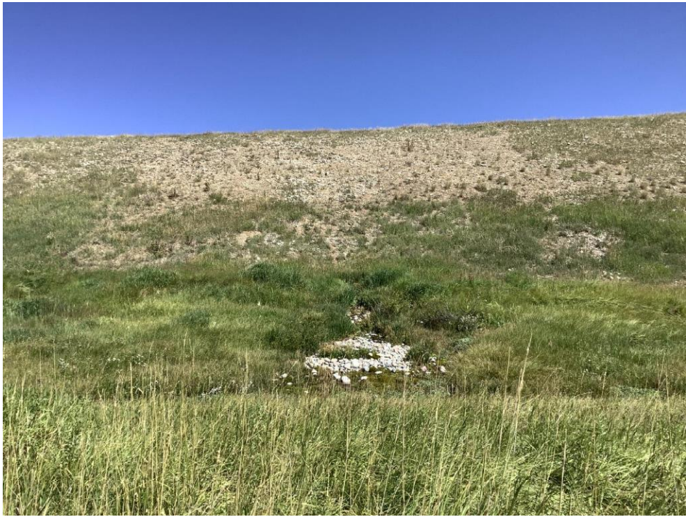
Photo 3-Looking east from Spring Location 3 at the toe of the bench, substantial flow was observed during the August 28 th field visit.
