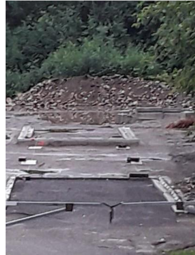
Figure 2: Standing Water at STT Site
