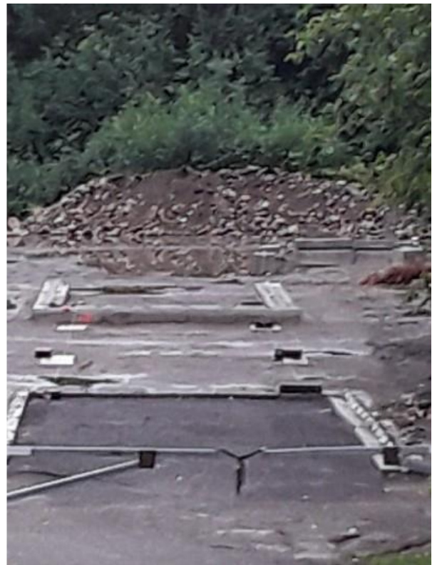
Figure 2: Standing Water at STT Site
