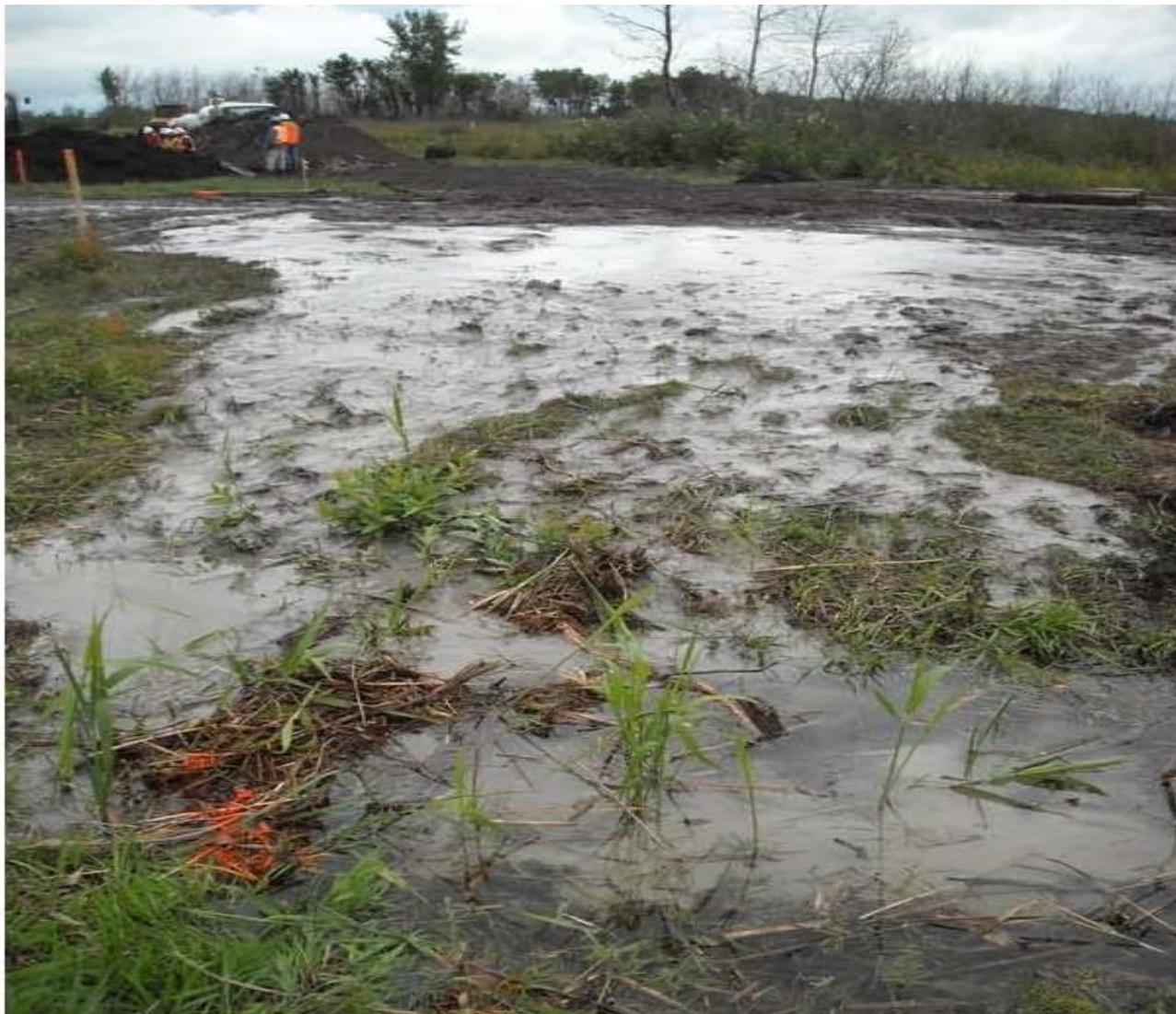
MP 845.70, Wetland W-845E and road surface frac-out, view southeast.
