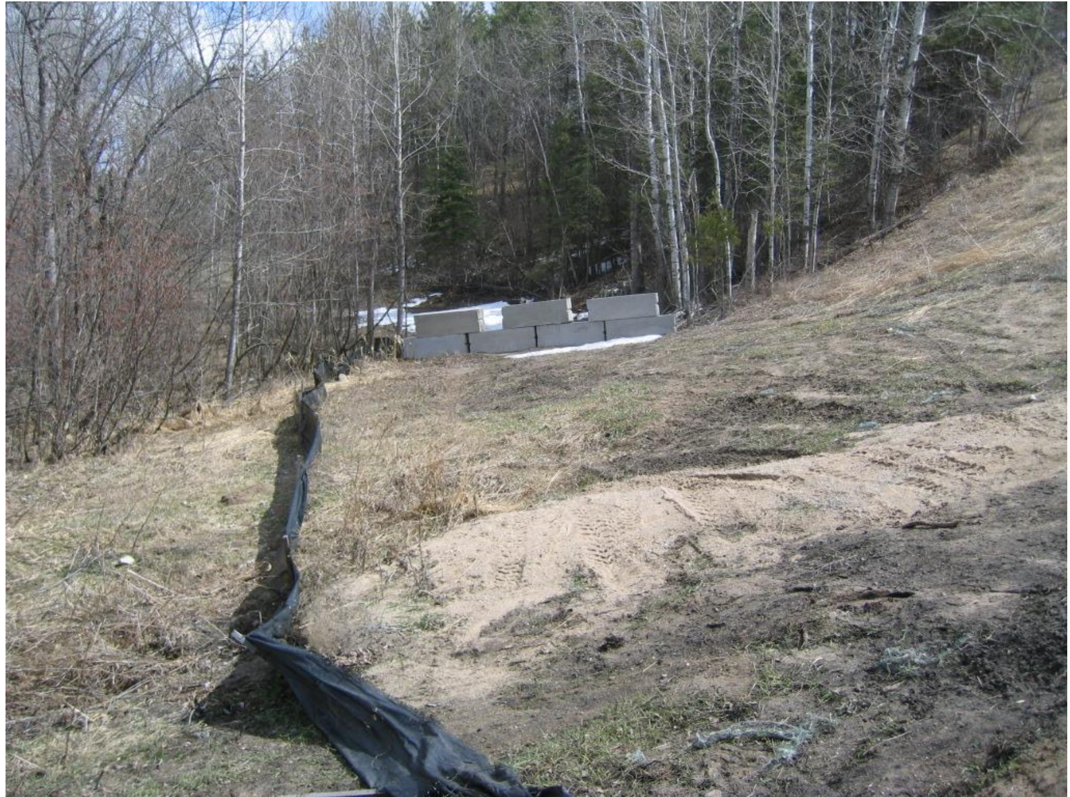
Clearwater River, bottom of E bluff. Cement barriers used to impede ATV access to the ROW after an access road was recently constructed for pipeline repair.
