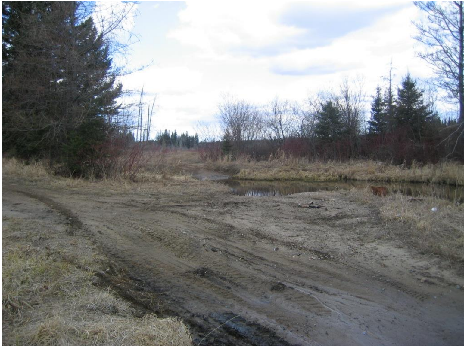
Close-up of Grant Creek pipeline corridor looking N toward OHV trail on railroad grade, indicating OHV off-trail destruction of stream banks and vegetation
