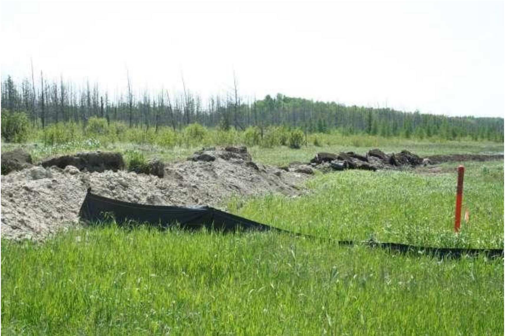
From W side ROW looking SE across transition from upland to wetland, Mud Lake.
