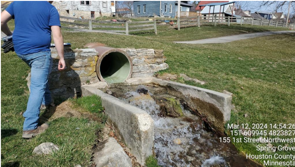
PHOTO NO. 3: View of water from pumping CW-1 entering the cascade aeration channel at sampling location SW-3.
