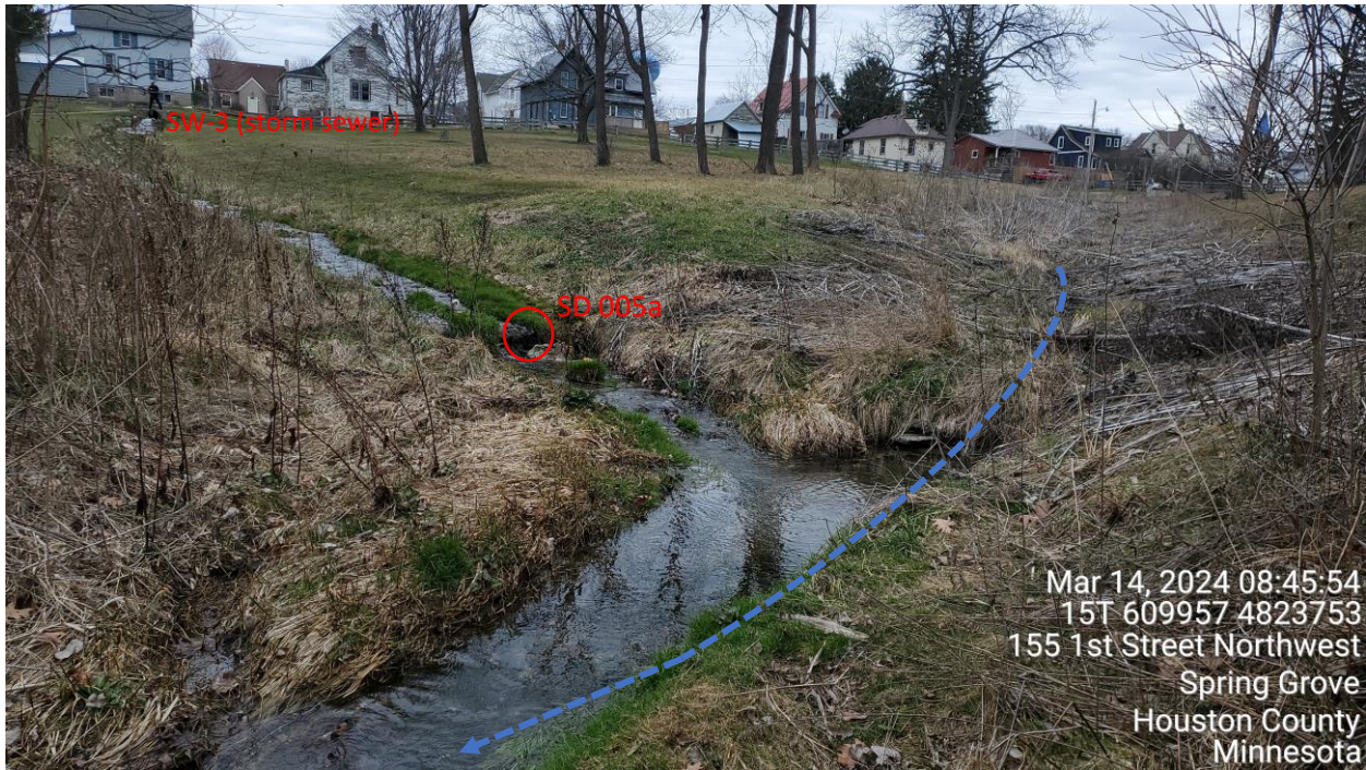
PHOTO NO. 5: Alternate view of the cascade aeration system discharge into the un-named stream channel, tributary to North Bear Creek. The natural intermittent stream would flow down from the background, toward the left of this photo. Station SD 005a is depicted.
