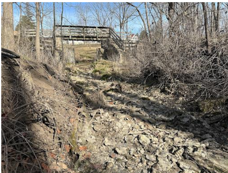
PHOTO NO. 9, bottom: Photo view faces upstream from a point just downstream of the trail bridge.
