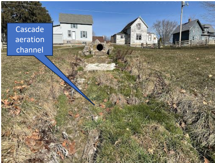
PHOTO NO. 8, middle: Without flow coming from CW-1, there was no flow exiting the storm sewer and the cascade aeration channel dried up.
