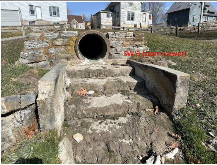
PHOTO NO. 7, top: Inspection of the CW-1 storm sewer outfall and cascade aeration system was conducted February 27, 2024 during a period when CW-1 was not pumping due to failure of the motor and pump stack.
