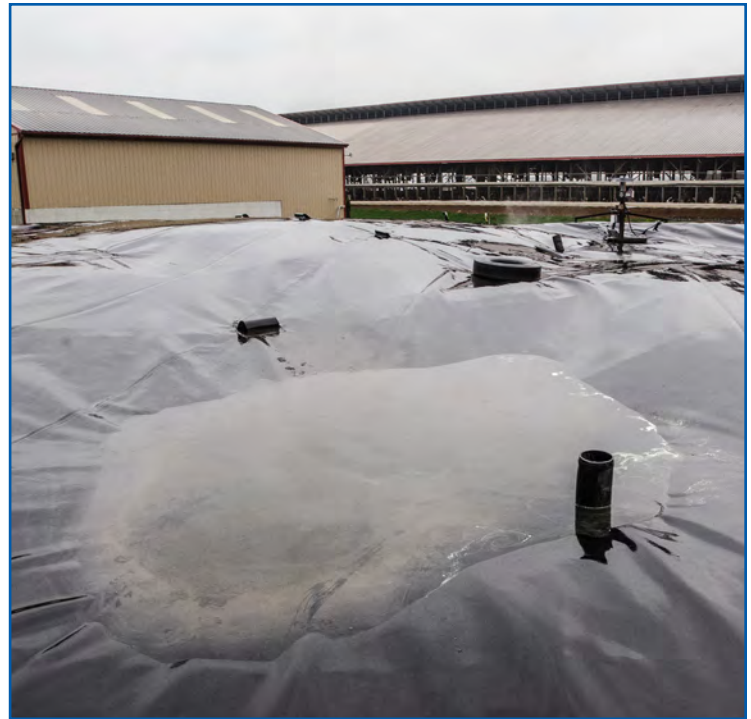
Rainwater and other debris collect in puddles on the cover of a manure lagoon located at a Pennsylvania dairy.
