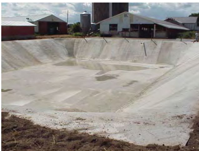
Figure 10D-3 Excavated animal waste storage pond with concrete liner ( Photo credit NRCS )
