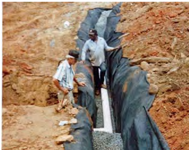
Figure 10D-28 Perforated collector pipe installed the gravel envelope with trench lined with geotextile
