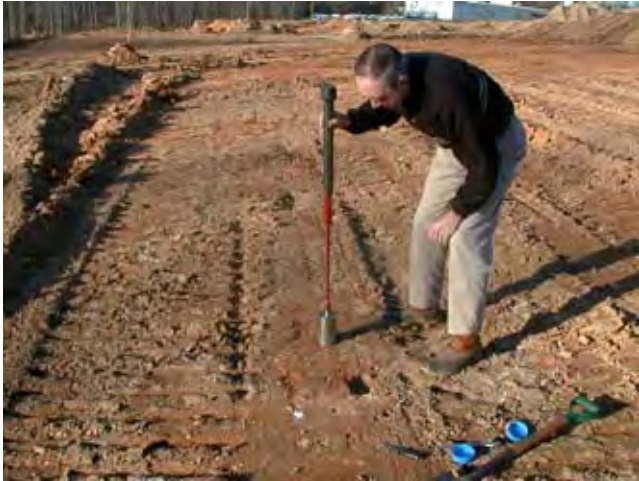
Figure 10D-33 Obtaining undisturbed sample of compacted clay liner using thin-walled drive cylinder
