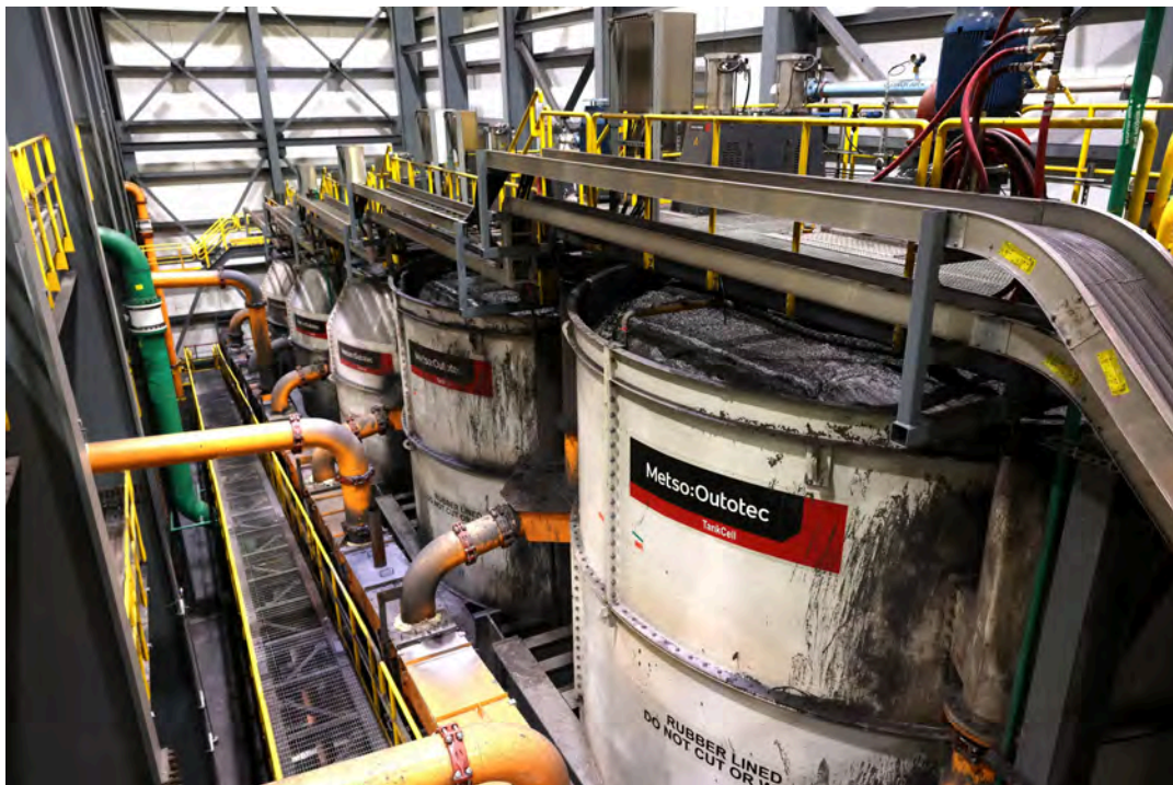
Flotation tanks remove silica from iron concentrate in the Keetac DR-grade pellet plant. Wyatt Buckner / Duluth Media Group
