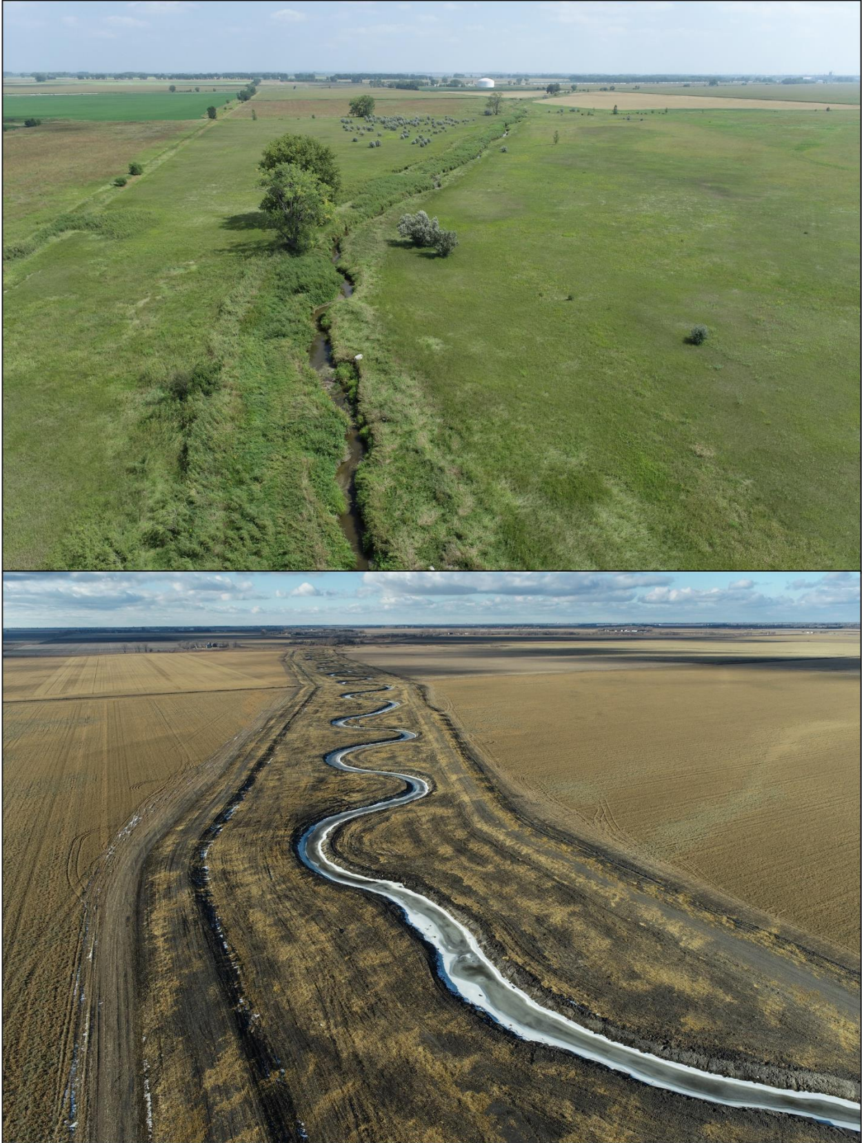
Figure 24. Pre- (top) and post-project (bottom) photos of the Stony Creek Restoration project (BRRWD 2025a).
