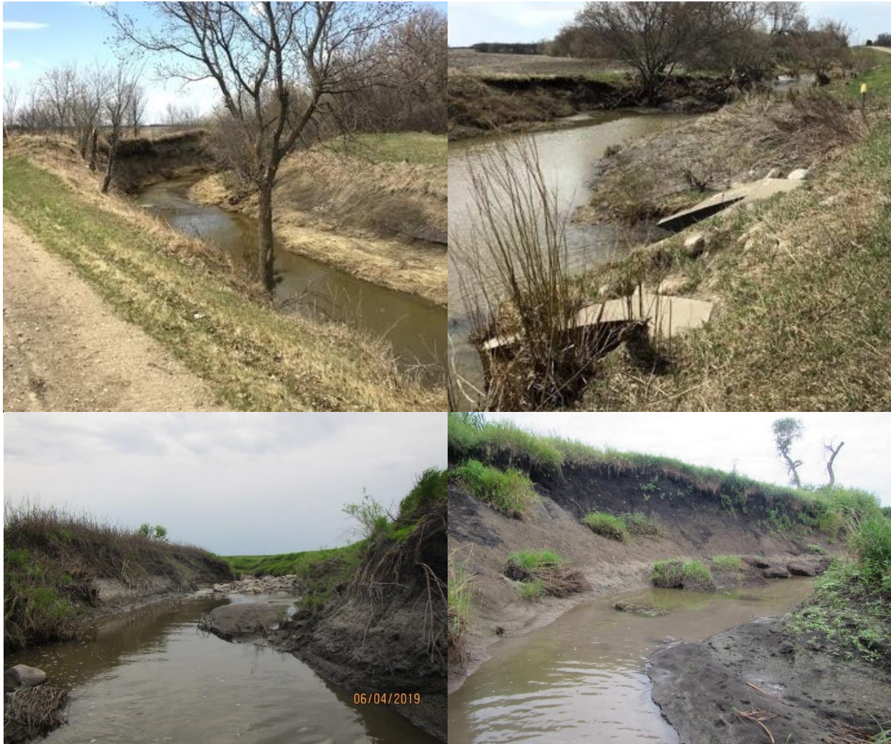
Figure 11. Bank erosion and instability documented in 2019 in Unnamed Creek (WID 09020104-516) along 240 th Street (top) and in Wolverton Creek (09020104-550) just downstream of 130 th Avenue South (bottom) (MPCA 2023a).
