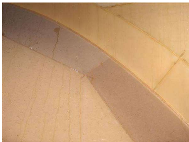
Figure 6 – ECTFE liner after 10 years of service
