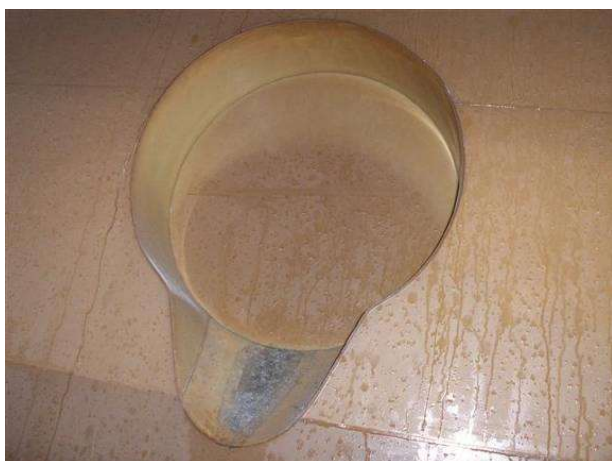
Figure 5 – ECTFE liner after 10 years of service
