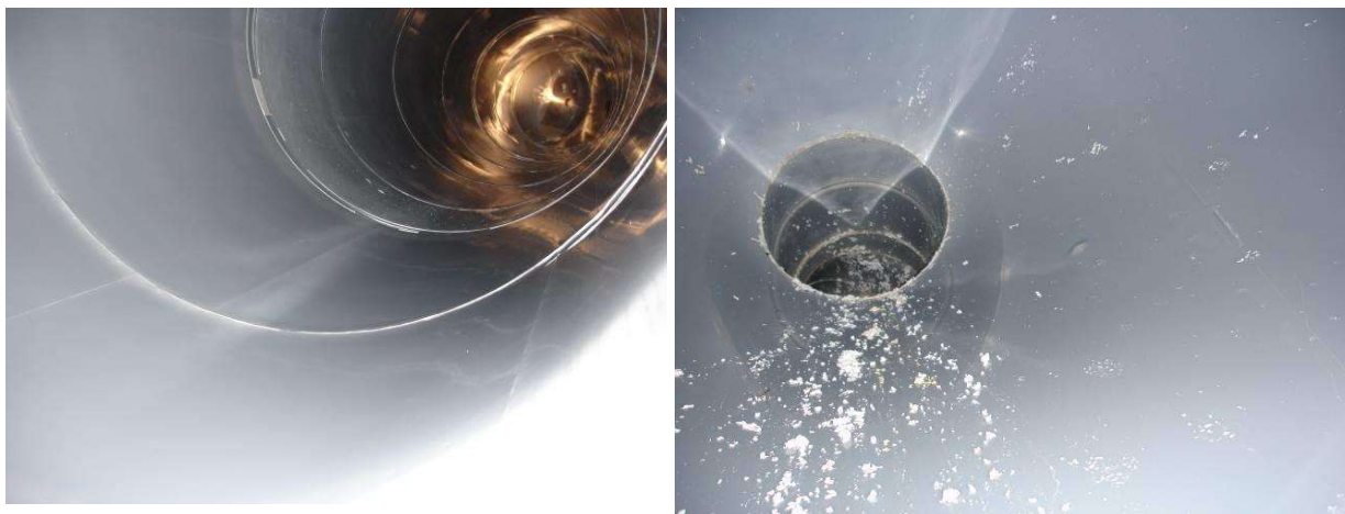
Figure 8: Inside view of the ECTFE liner
