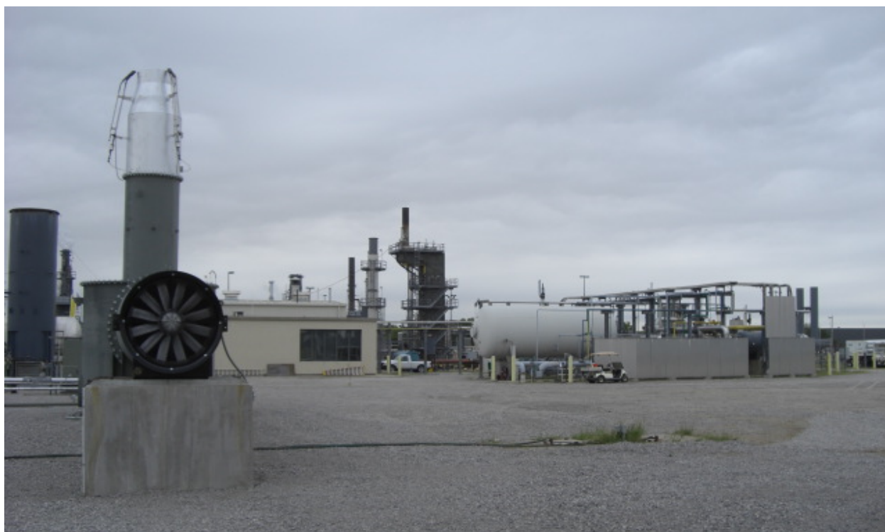
Figure 4-1. Overall View of Flare Test Facility
