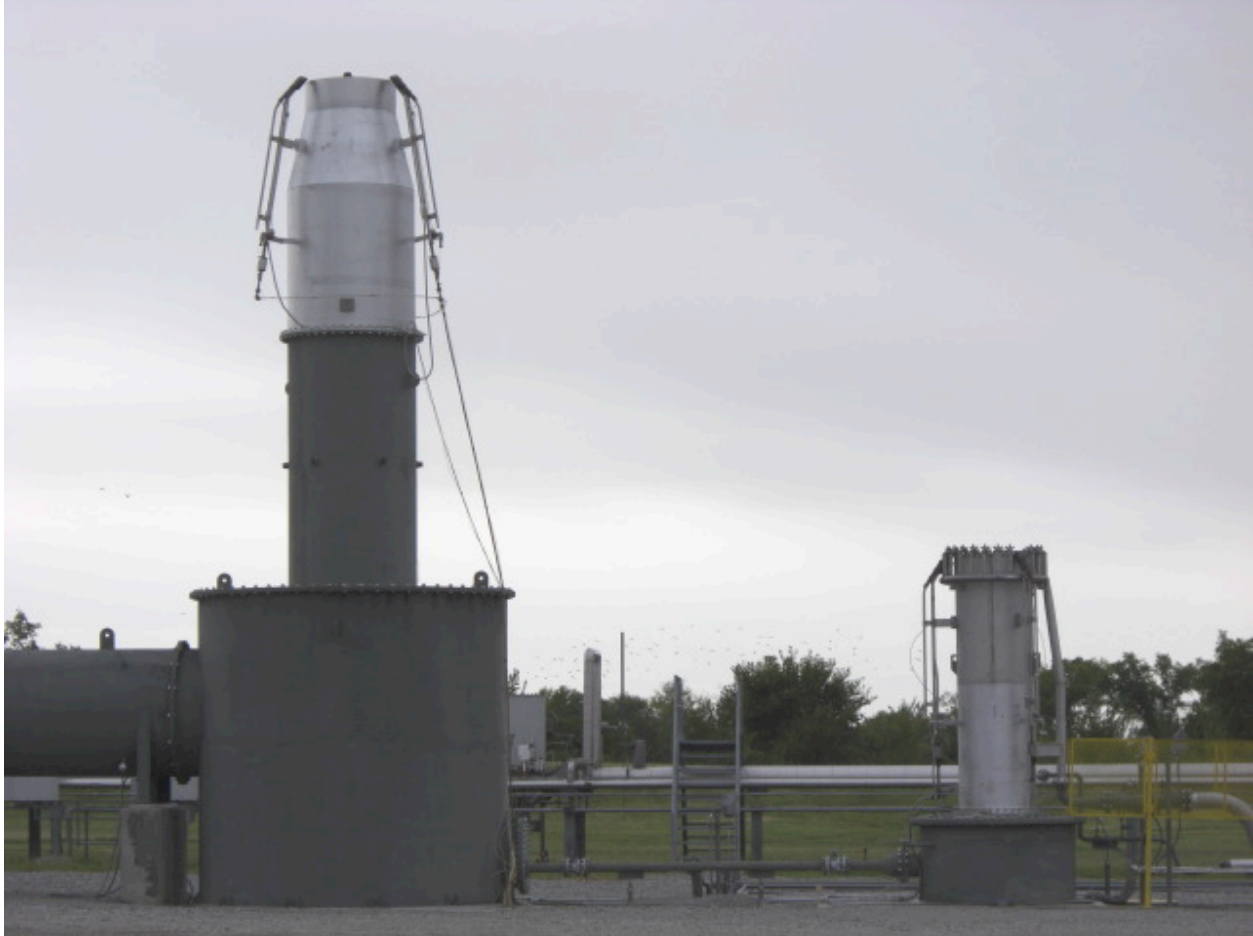
Figure 2-1. Flare Burners Used in Study. Air Flare John Zink Model LHTS-24/60 (left) and Steam Flare John Zink Model EE-QSC-36" Flare Tip (right) used in the study
