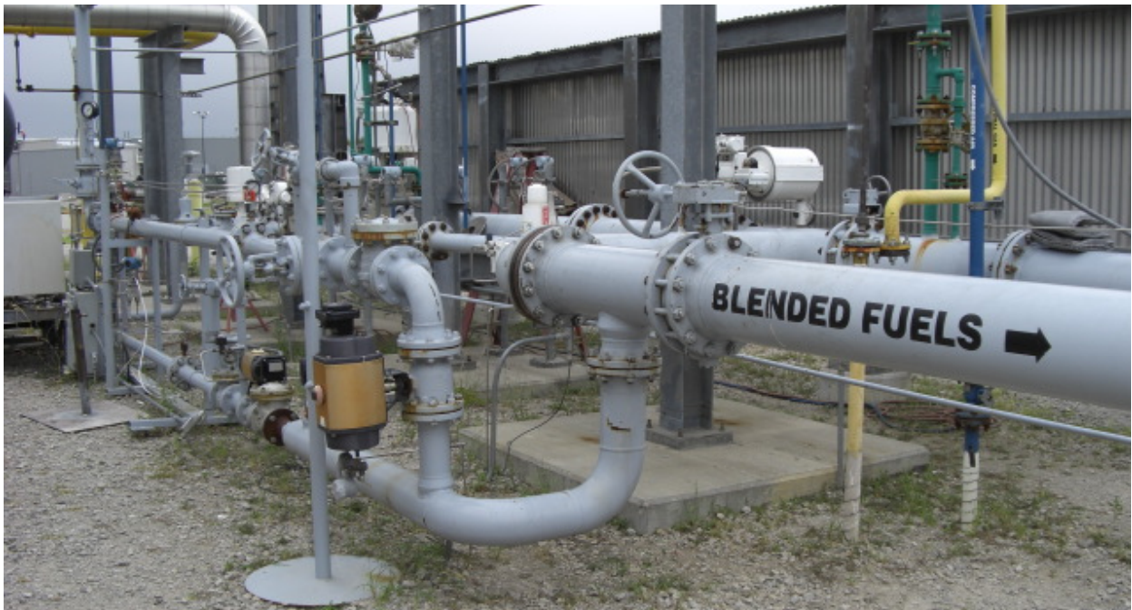
Figure 4-4. Vent Gas Supply. Piping for flow control, mixing and measurement of the vent gas supply
