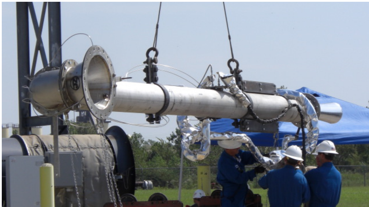
Figure 4-8. Sample Collector at Near Ground Level. Collector inlet is at foreground and eductor is at far end. In photo, Zink personnel make adjustments to heated transfer line supports. Shackles and cable at center allow crane to lift and position Sample Collector.
