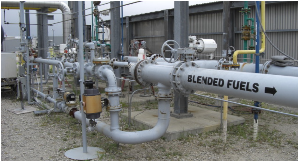
Figure 4-4. Vent Gas Supply. Piping for flow control, mixing and measurement of the vent gas supply
