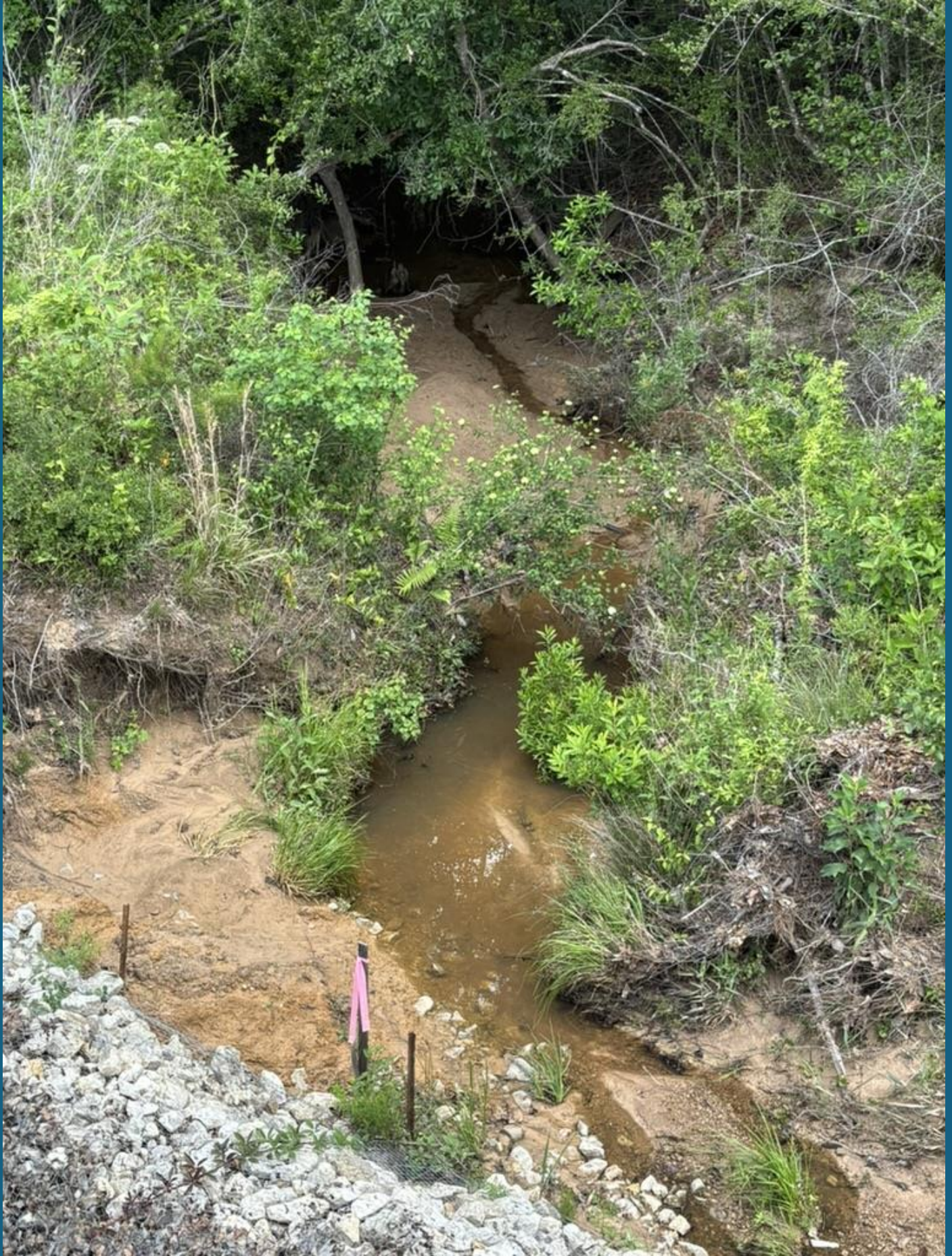
Sedimentation on private property 4-20-2026 Creek is now a stream due to sediment.
