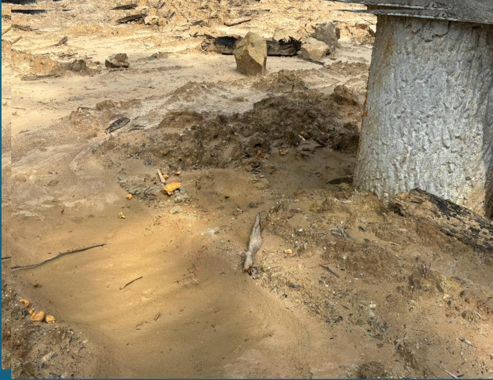
5-8-2026 Village Creek Bike Trail Expansion Joint Trash
