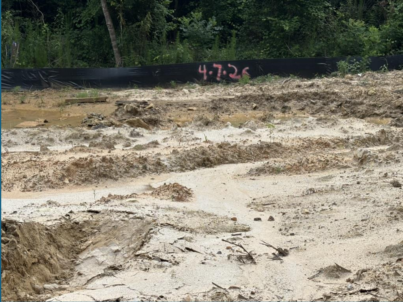
5-31-2026 Concrete dregs remaining Village Creek Bike Trail
