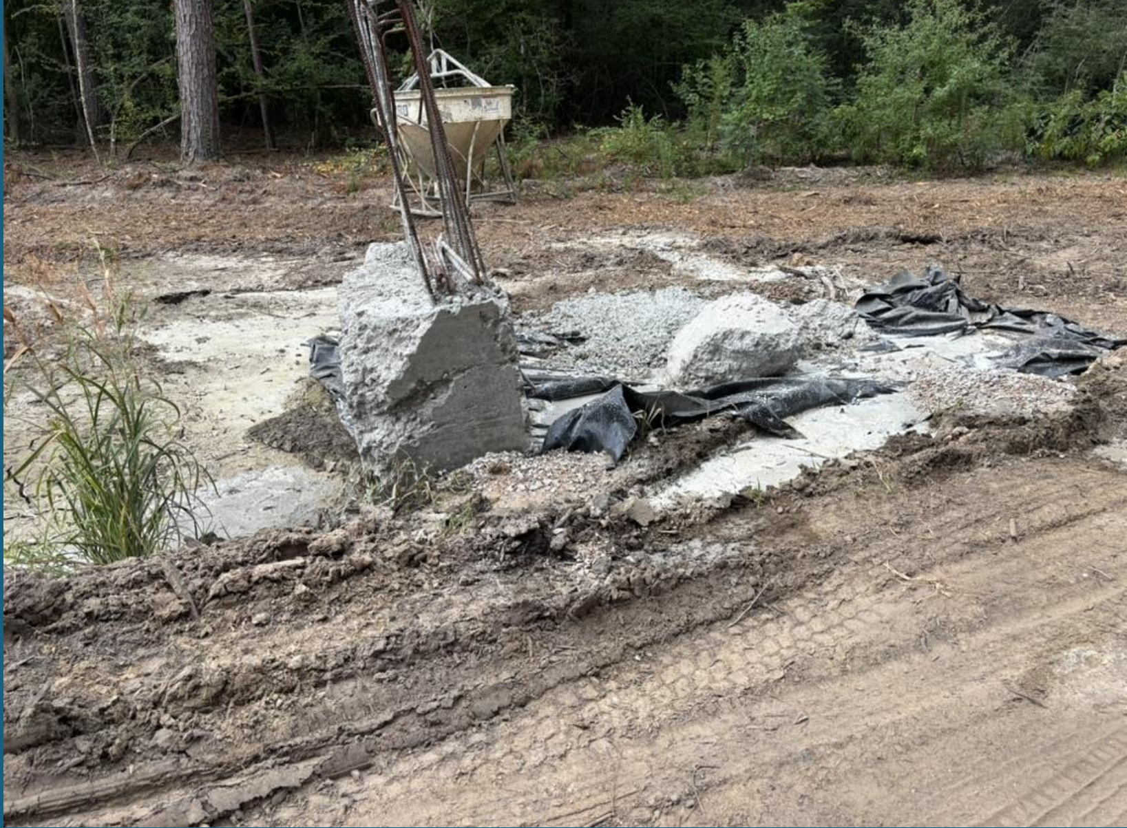
8-1-2026 Village Creek Bike Trail south side concrete wash out
