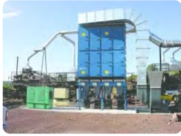
DLMC 4/8/15 Baghouse Dust Collector Rock Crushing
