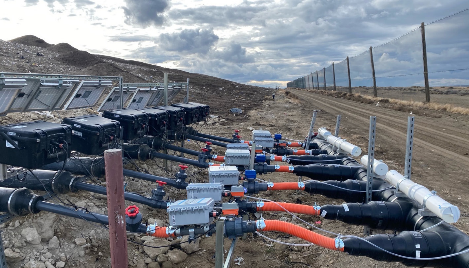
Horizontal gas collectors with real-time tech at a landfill. Photo Source: LoCI Controls.
