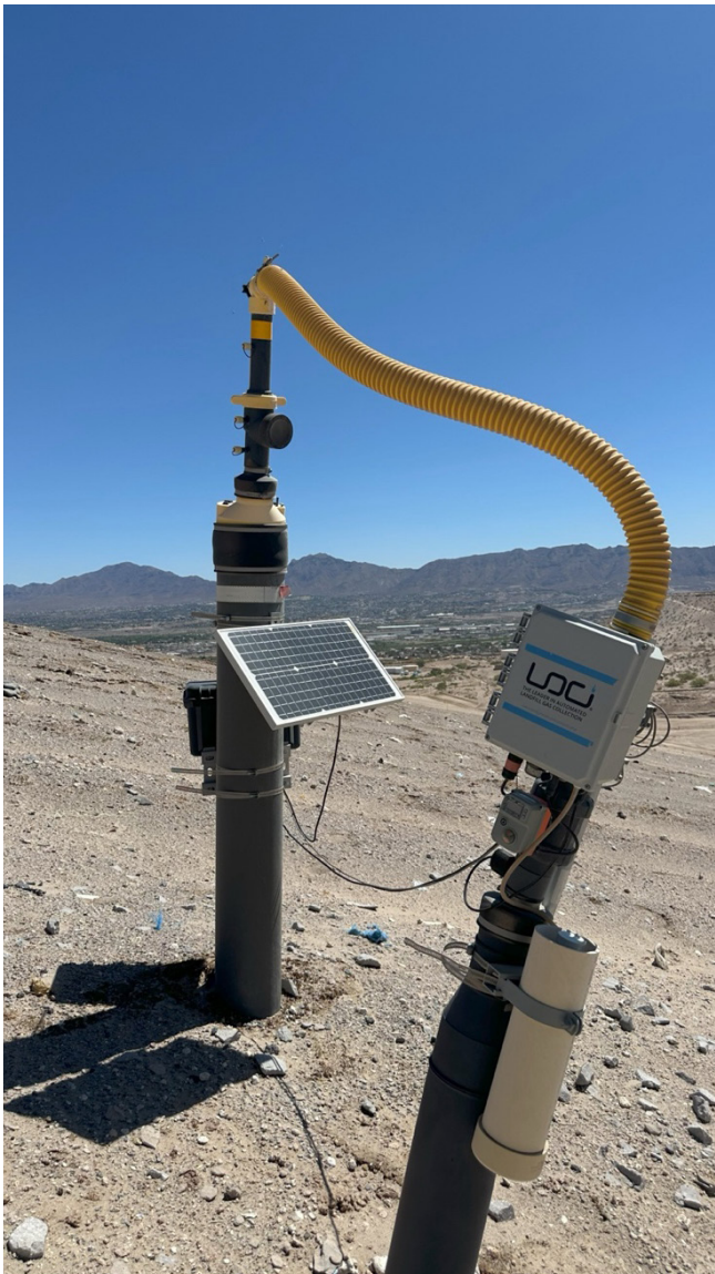
A vertical wellhead with real-time tech at a landfill. Photo Source: LoCI Controls.
