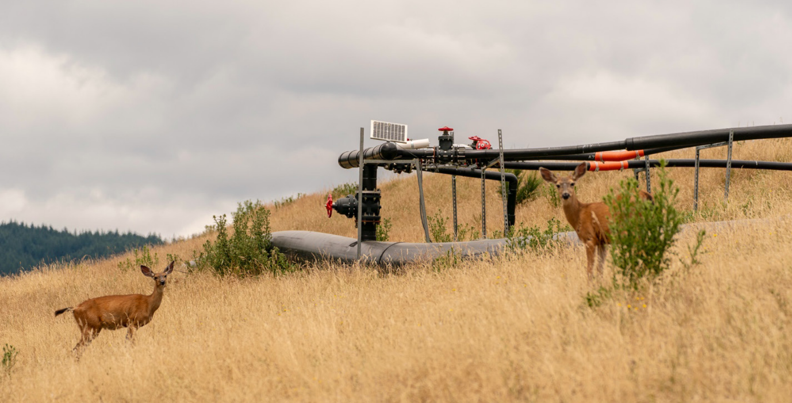
A landfill wellhead with real-time monitoring and automated tuning technology. Photo Source: LoCI Controls.
