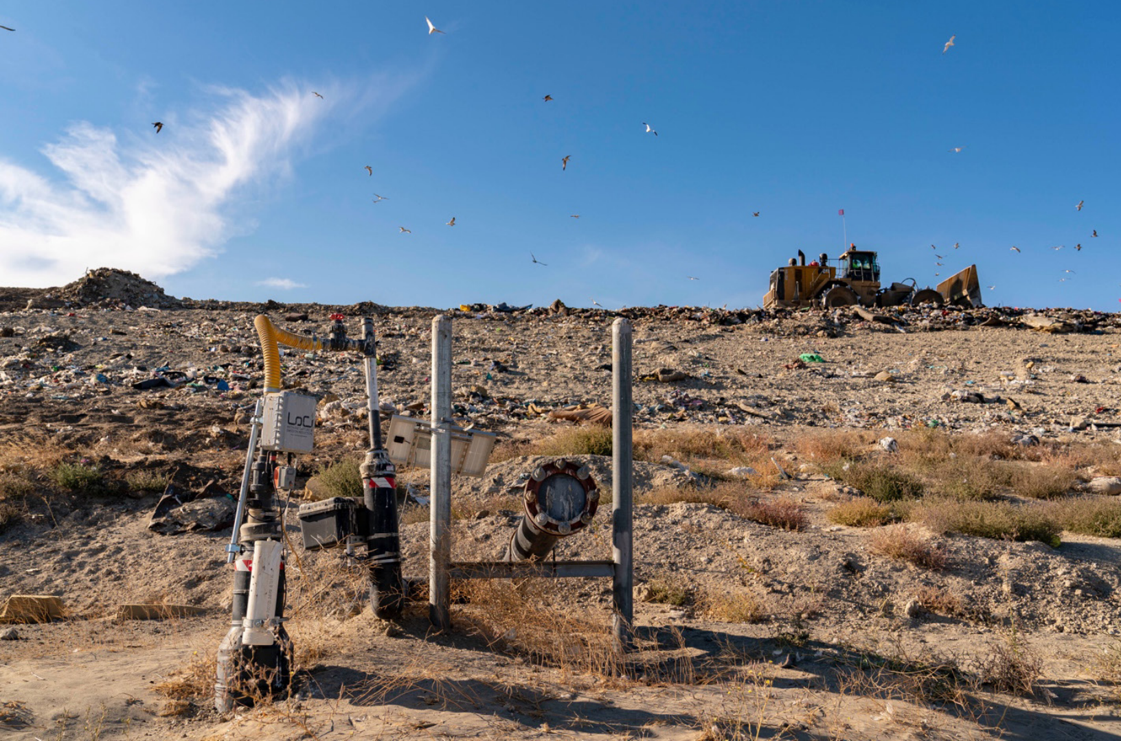
A horizontal gas collector with real-time tech at a landfill working face. Photo Source: LoCI Controls.
