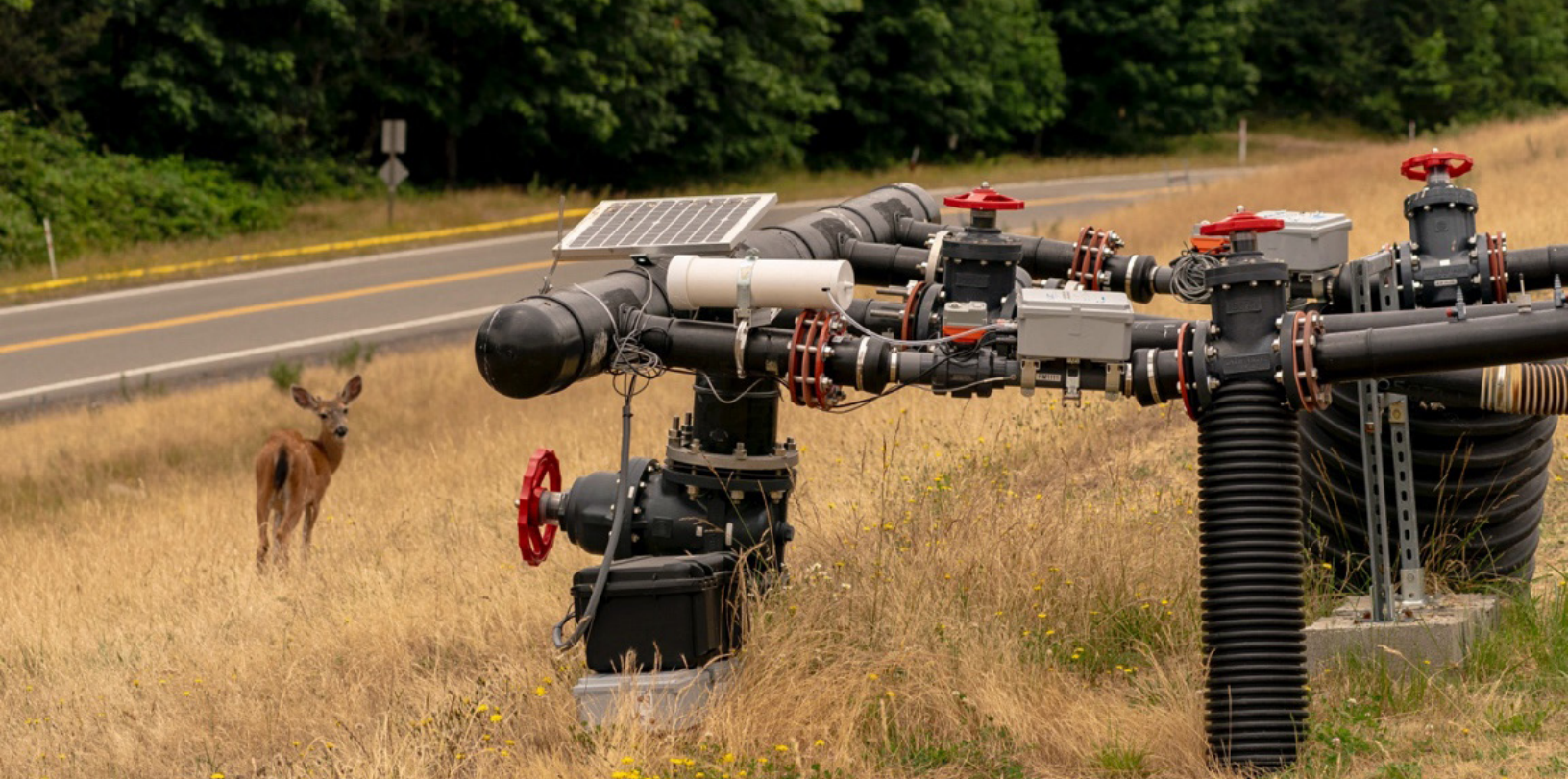
A landfill wellhead with real-time tech. Photo Source: LoCI Controls.
