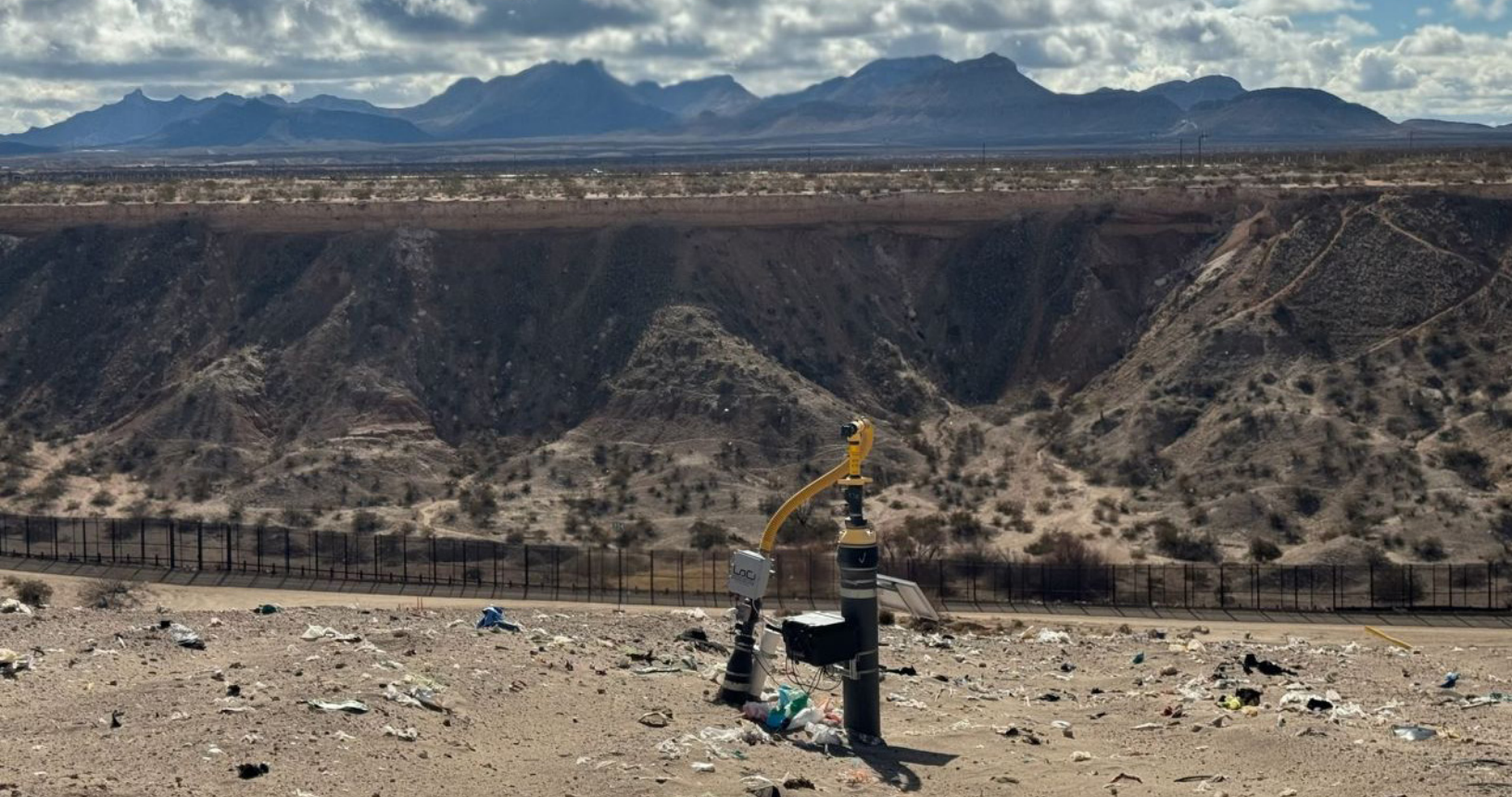
A vertical landfill wellhead with real-time tech. Photo Source: LoCI Controls.
